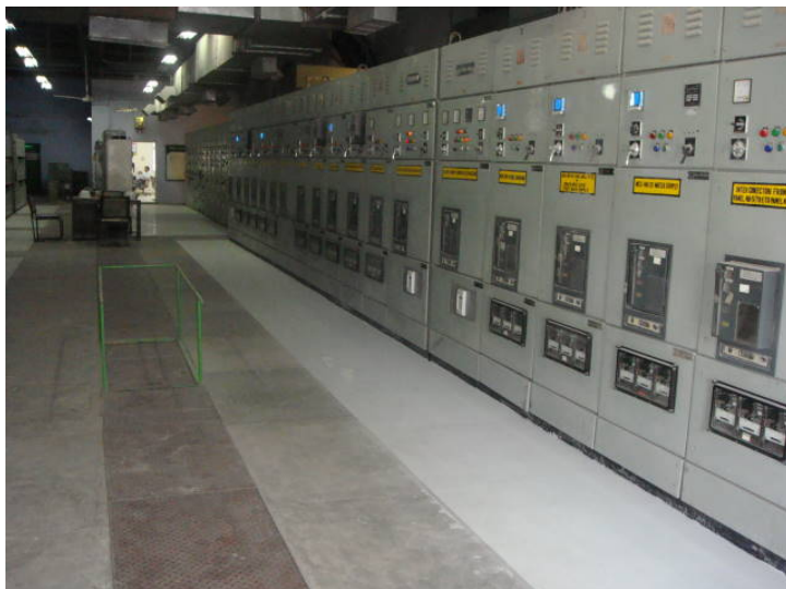
Dielectric Floor Coating in Front of HV Control Panels
