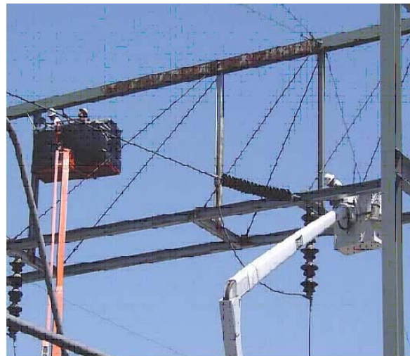
Bus Bar Coating
