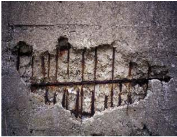
Concrete Cancer – Loss of Alkalinity; Spalling ; Re-Bar Corrosion;
