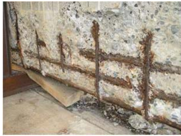
Severe Concrete Corrosion
