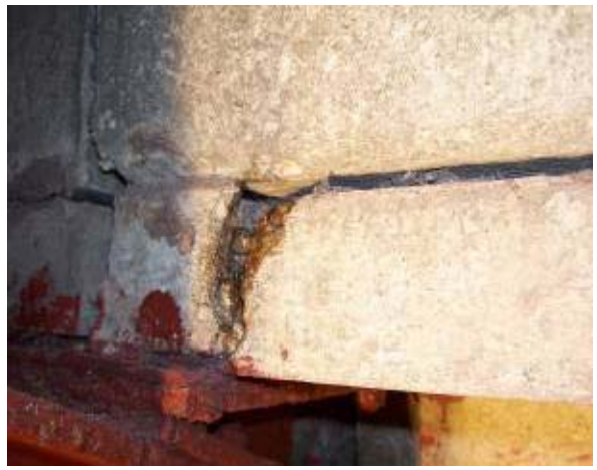
Sulfuric Acid Attacked Concrete
