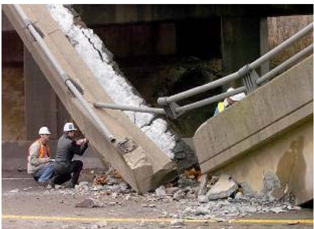
Catastrophic Concrete Corrosion & Failure
