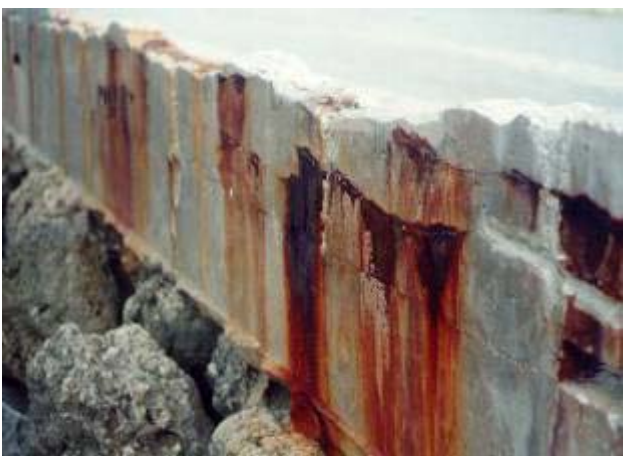
Severe Corrosion in Concrete
